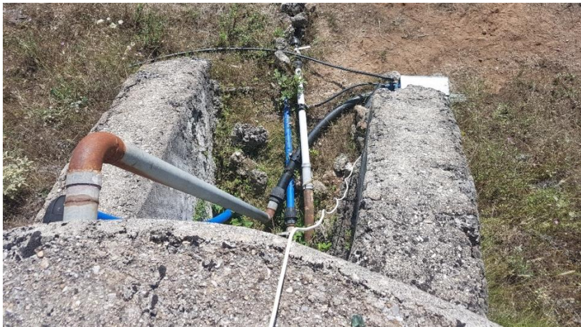
Figure 4-43: Example of drinking water piping
